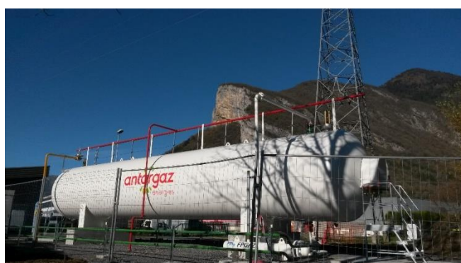
Cuve propane 70 m3 _ 31 Tonnes
