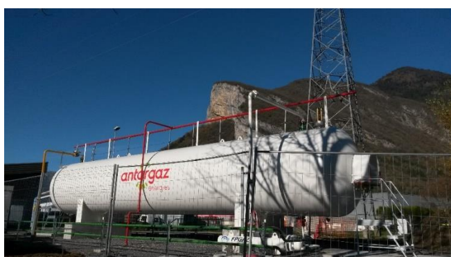
Cuve propane 70 m3 _ 31 Tonnes
